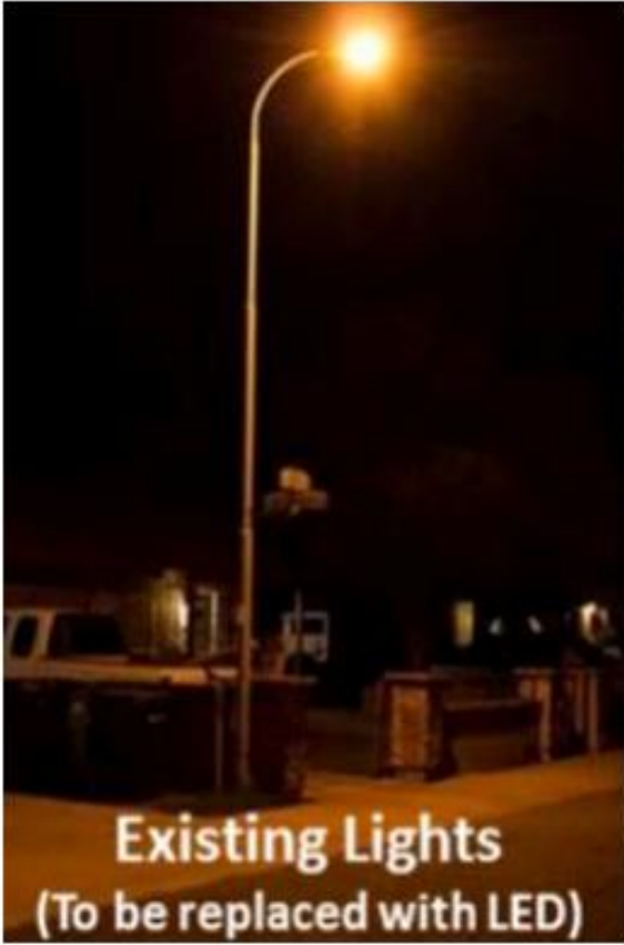
Existing 2200 Kelvin HPS
